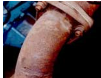
Fig. 3-6 Damaged Exhaust System
